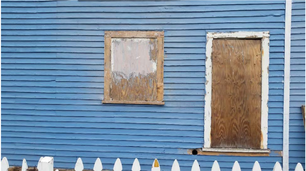
622 Deery St. – Close-up of boarded window openings on SE elevation
