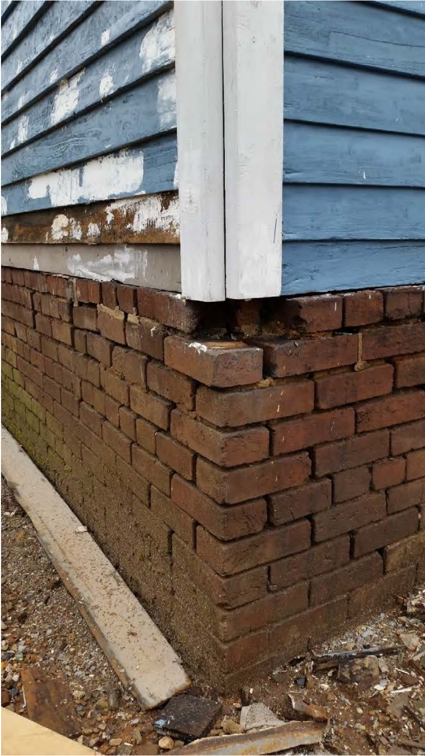
622 Deery St. – Brick foundation to be repointed
