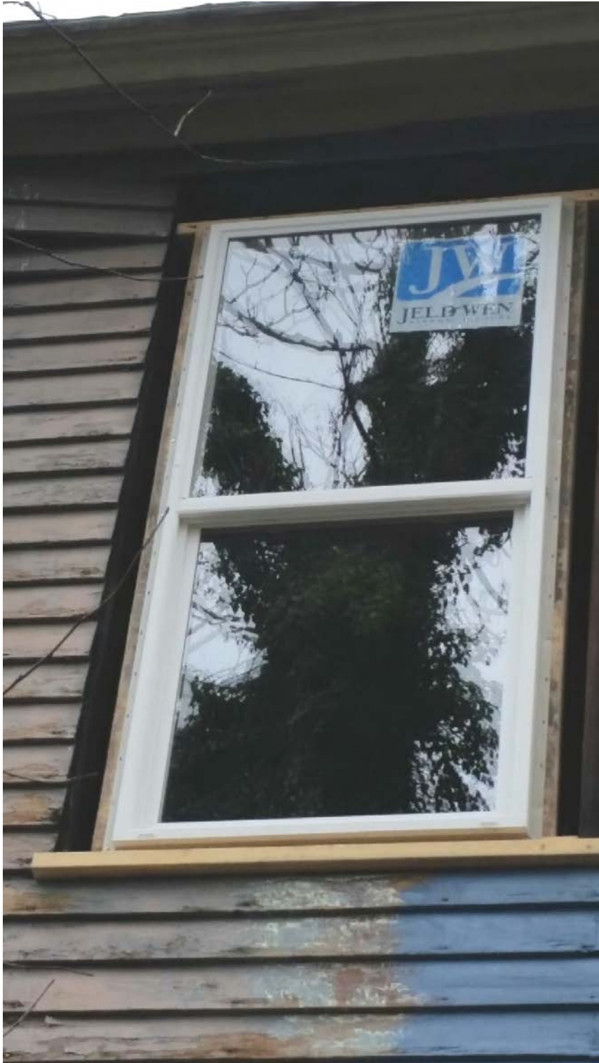
622 Deery St. – New vinyl window on 2 nd level – NW side
