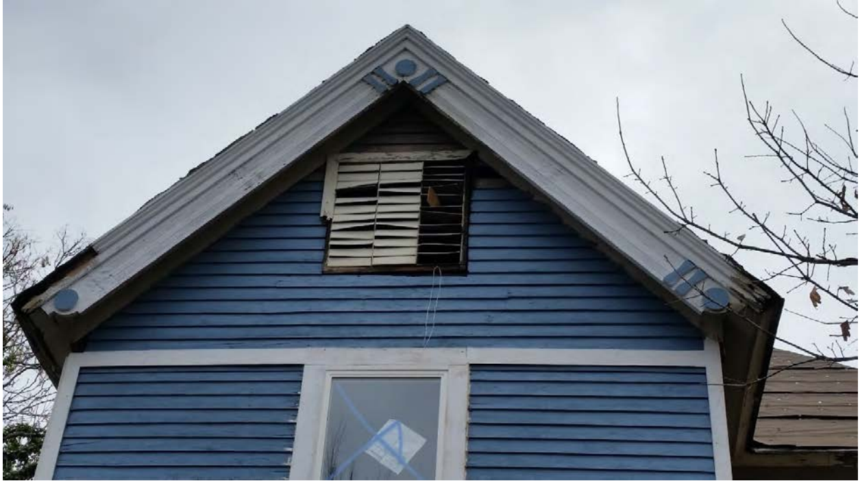
622 Deery St. – Louvered attic vent to be repaired or replaced
