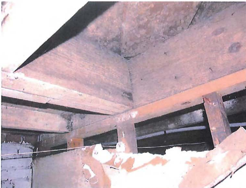
Triple beam framing into girder that supports the front brick façade. Wall not adequate to support load.
