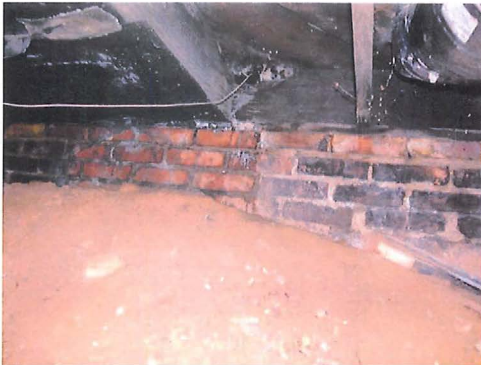
Rim joist is wet, indicating water penetration from outside. Joists connection is being lost.
