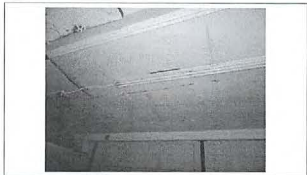
Subject Ceiling discoloration Viewing Interior
