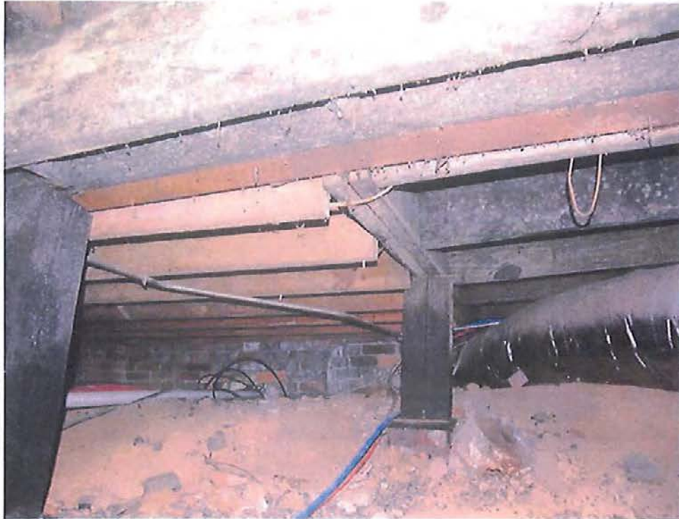
New joists replaced original joists. New joists connection failed.
