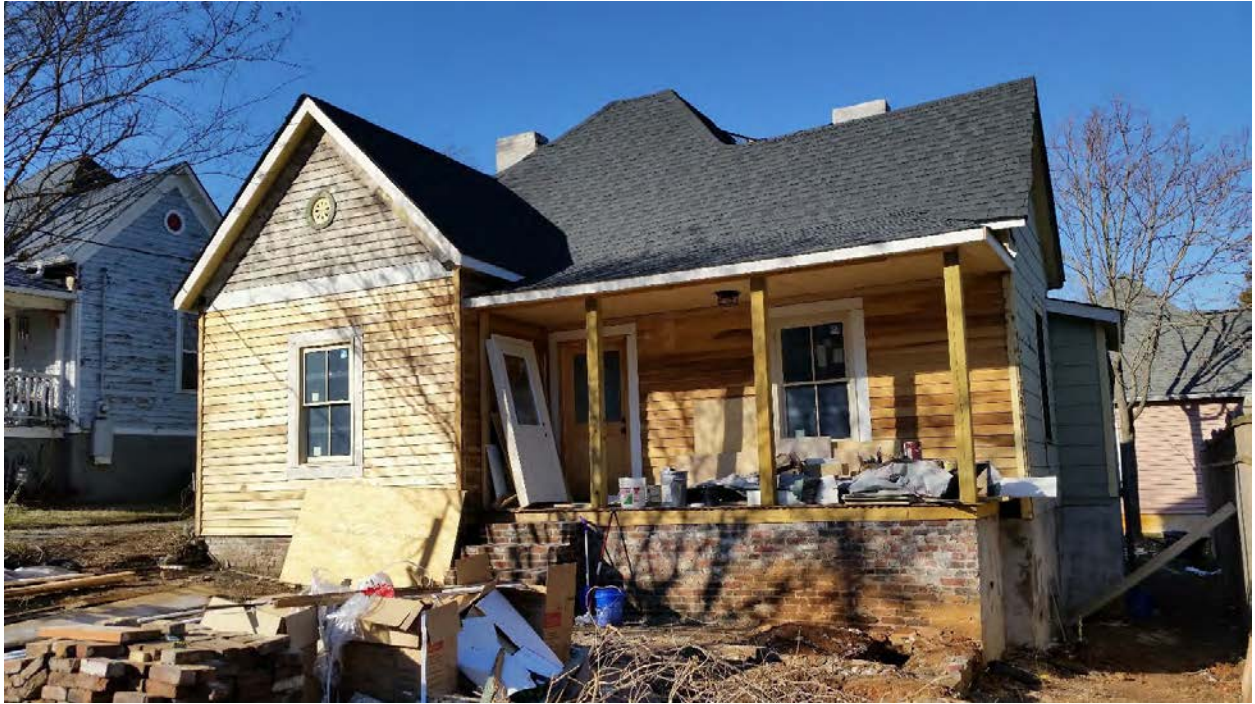
227 Leonard Place – Front façade – in progress – rear roof addition is barely visible.
