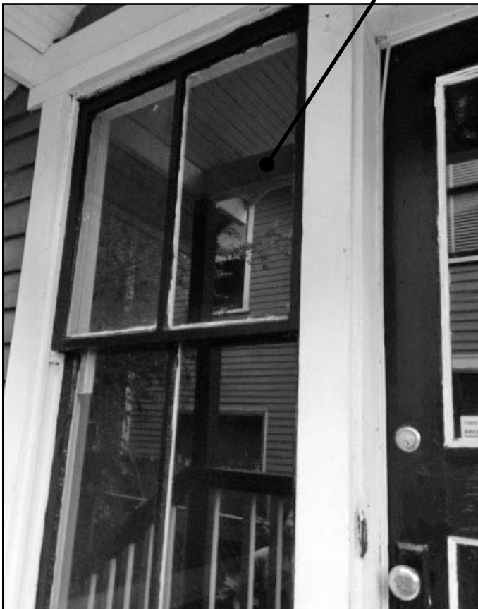
First level toward rear: Non-original window and door
