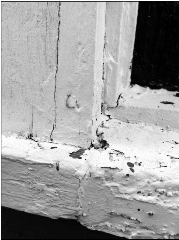
Original Window: First level on front gabled portion, rotten frame & sash
