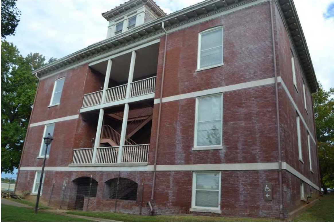
Duncan Law School – South side showing late-added fire escape in open balcony area
