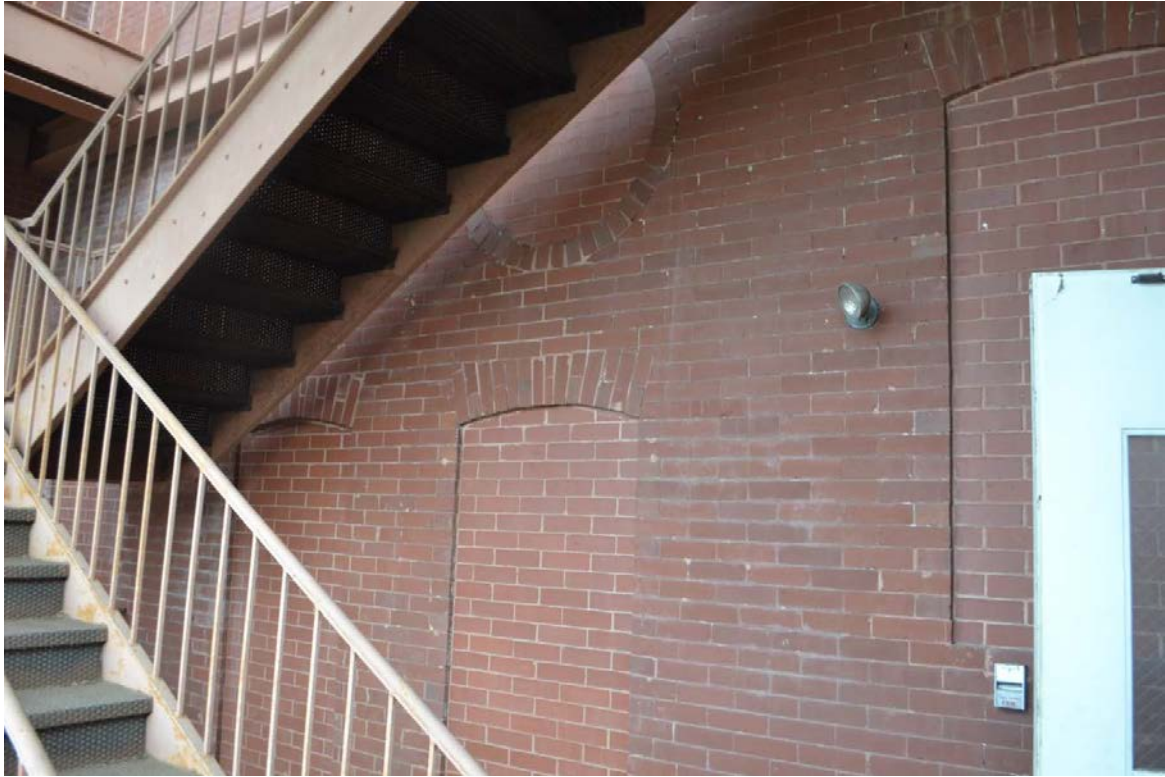
Duncan Law School – Fire escape (to be removed) in atrium space showing brick-infilled windows
