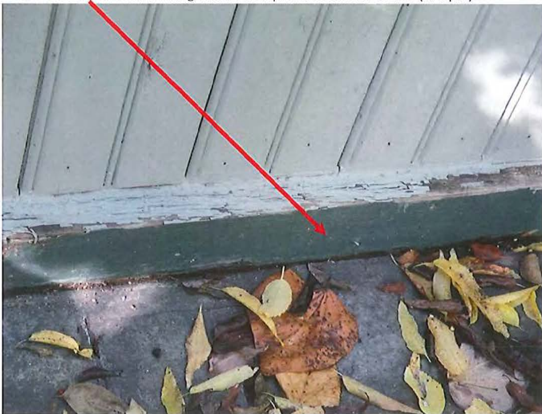
Below: wood trim in contact with ground to be replaced with Azek PVC trim (or equal).
