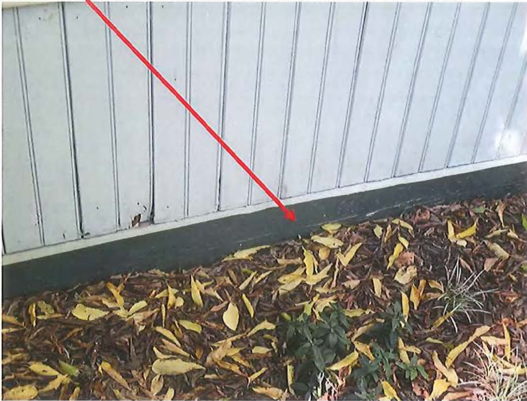
Below: wood trim in contact with ground to be replaced with Azek PVC trim (or equal).
