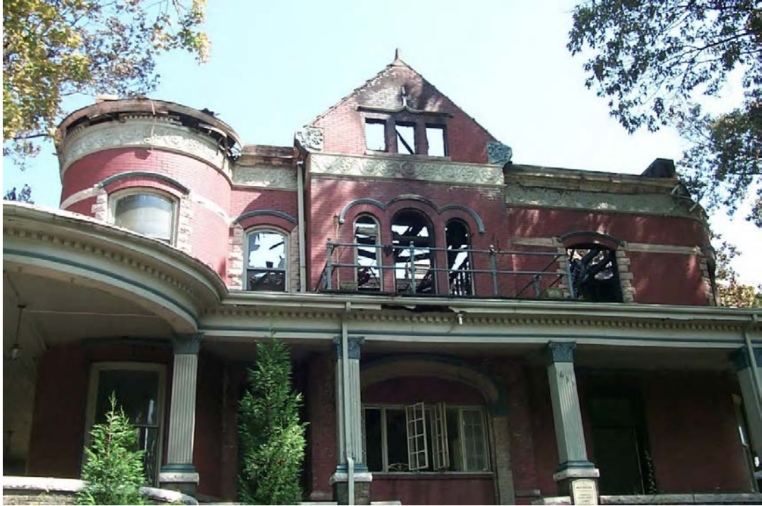
1633 Clinch Ave. – After burn
