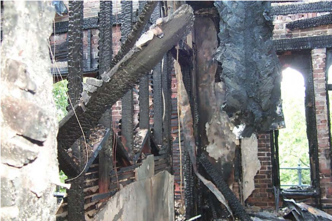
1633 Clinch Ave. – After burn
