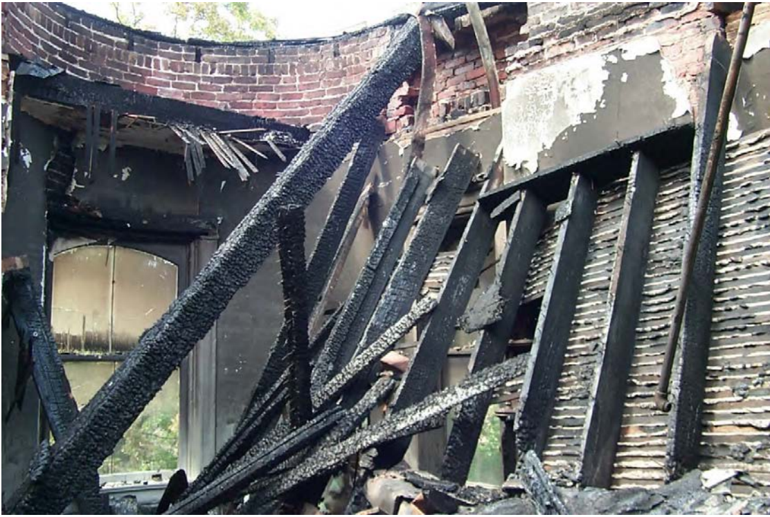
1633 Clinch Ave. – After burn
