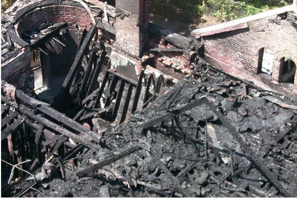
1633 Clinch Ave. – After burn
