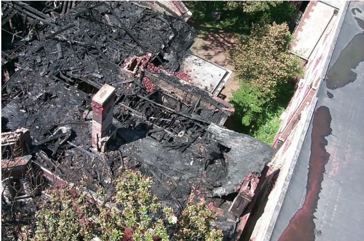
1633 Clinch Ave. – After burn
