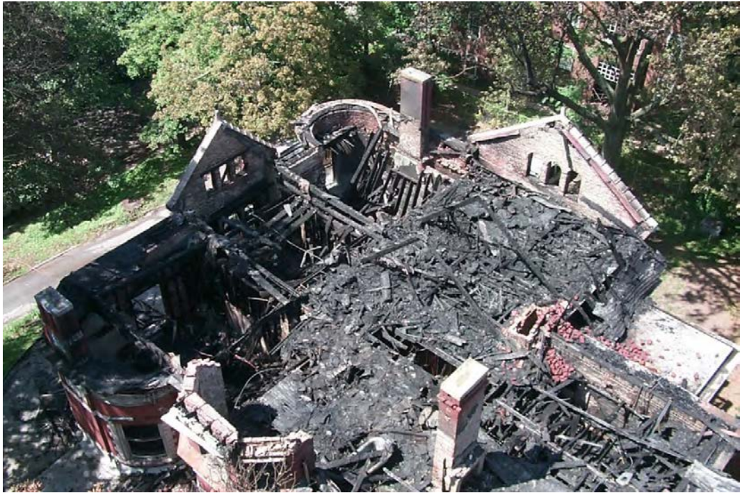
1633 Clinch Ave. – After burn
