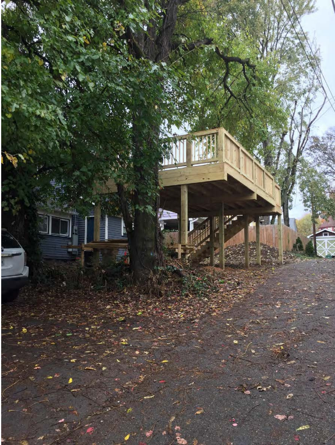
706 Luttrell – From 3 rd Street looking north up the alley. The deck is 5' from the property line or existing retaining wall near the large tree and the nearest post in picture is 7' from the alley.
