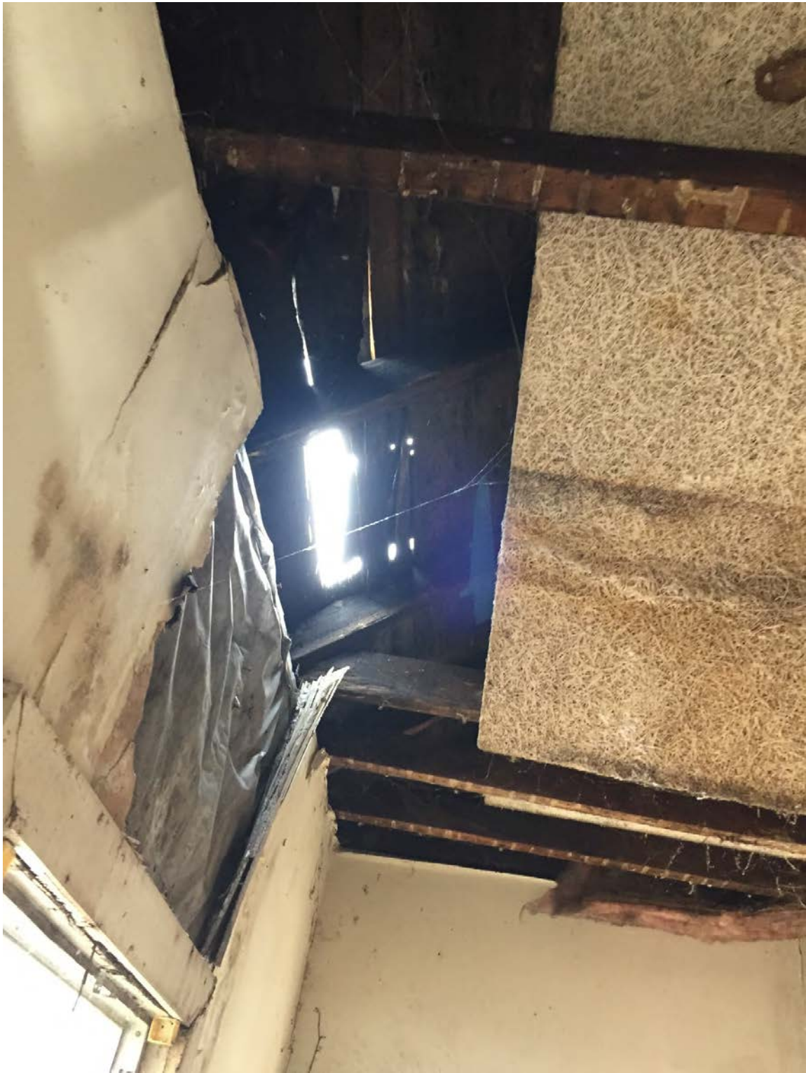
219 Twelfth – Looking up at hole in roof, 2
