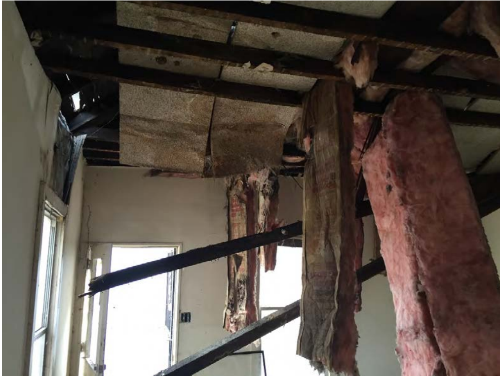
219 Twelfth – Interior view showing fallen floor joists
