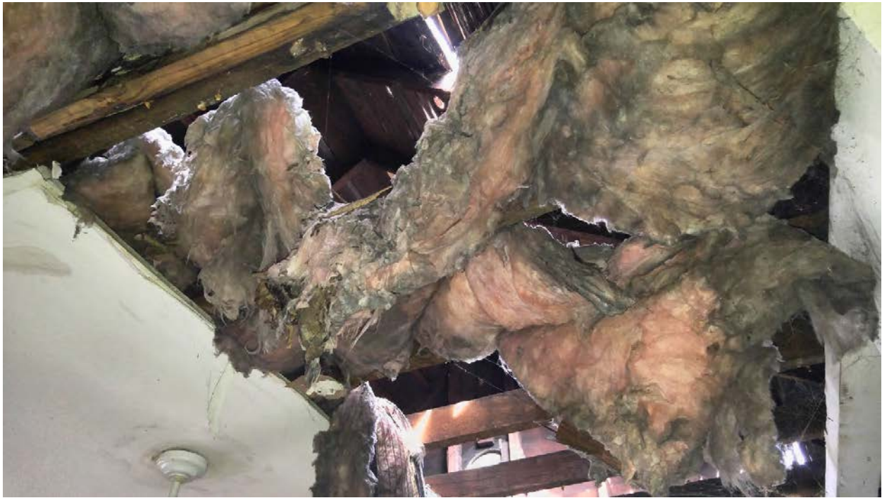
219 Twelfth – Looking through ceiling at large hole in roof
