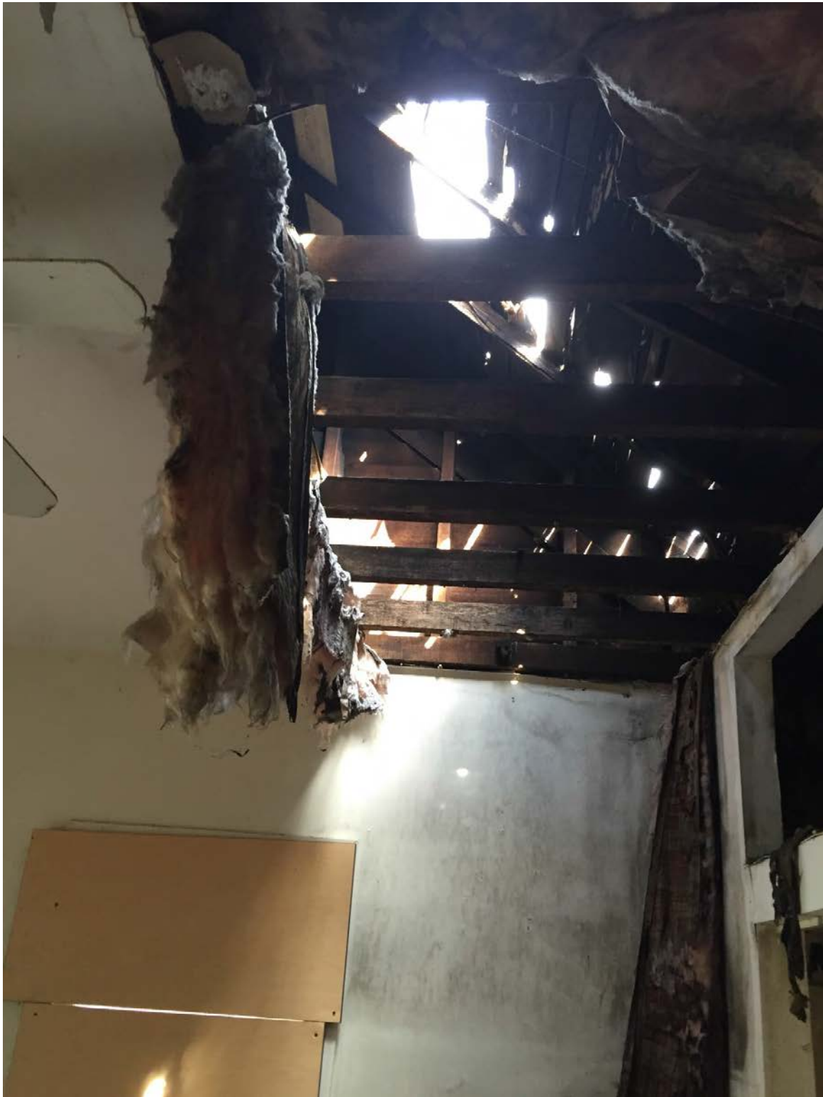
219 Twelfth – Looking up at hole in roof, 1
