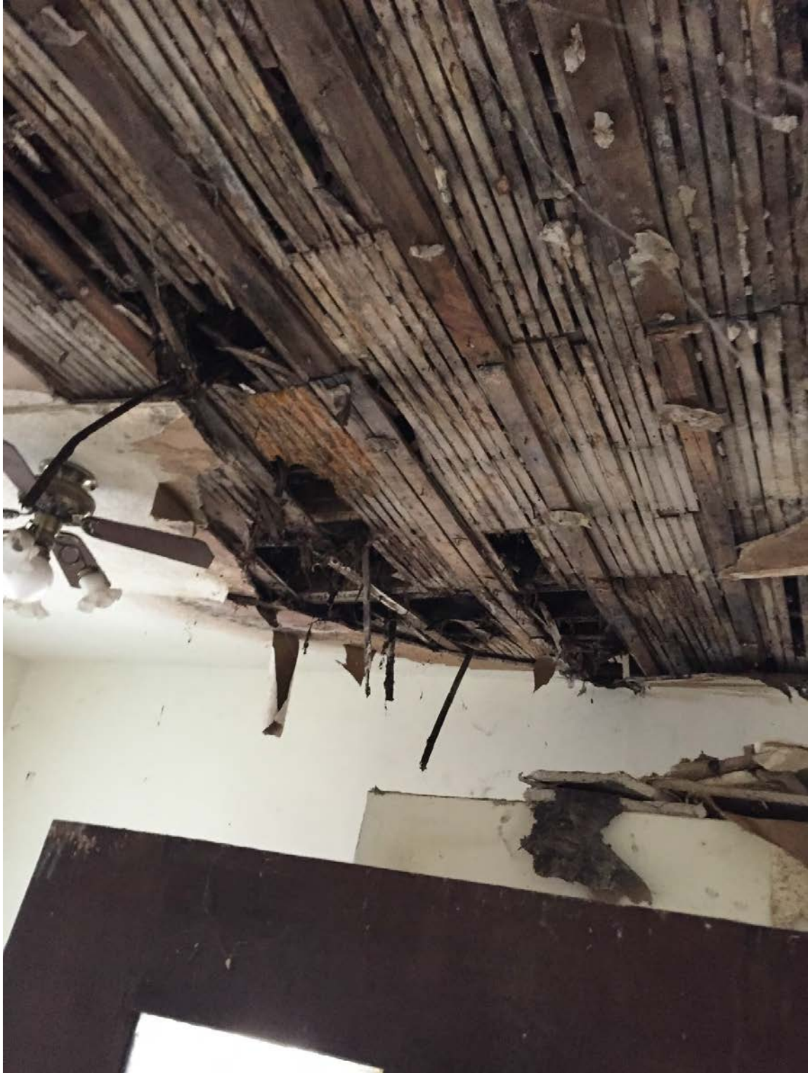
219 Twelfth – 2 nd level looking up at fallen ceiling lathe
