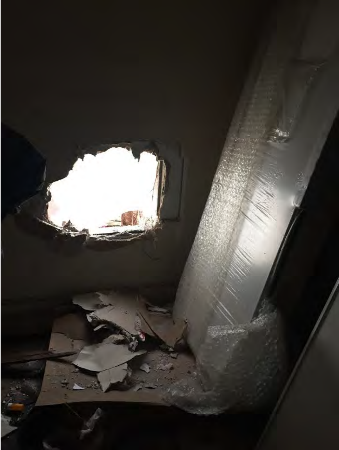
219 Twelfth - Hole in wall from interior
