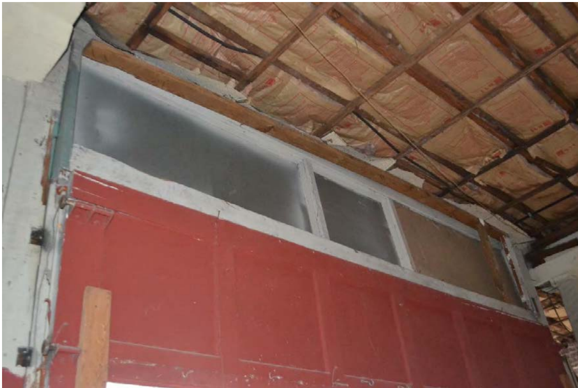
116 E. Jackson -- Overhead garage door from interior -- to be replaced with storefront
