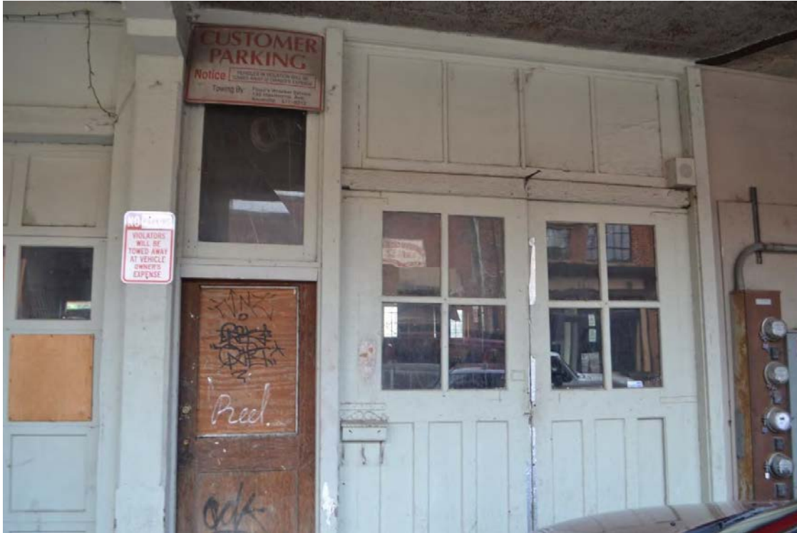
116 E. Jackson Ave. - Existing overhead garage door to be replaced with storefront (left) and side-opening carriage doors with transom (right)
