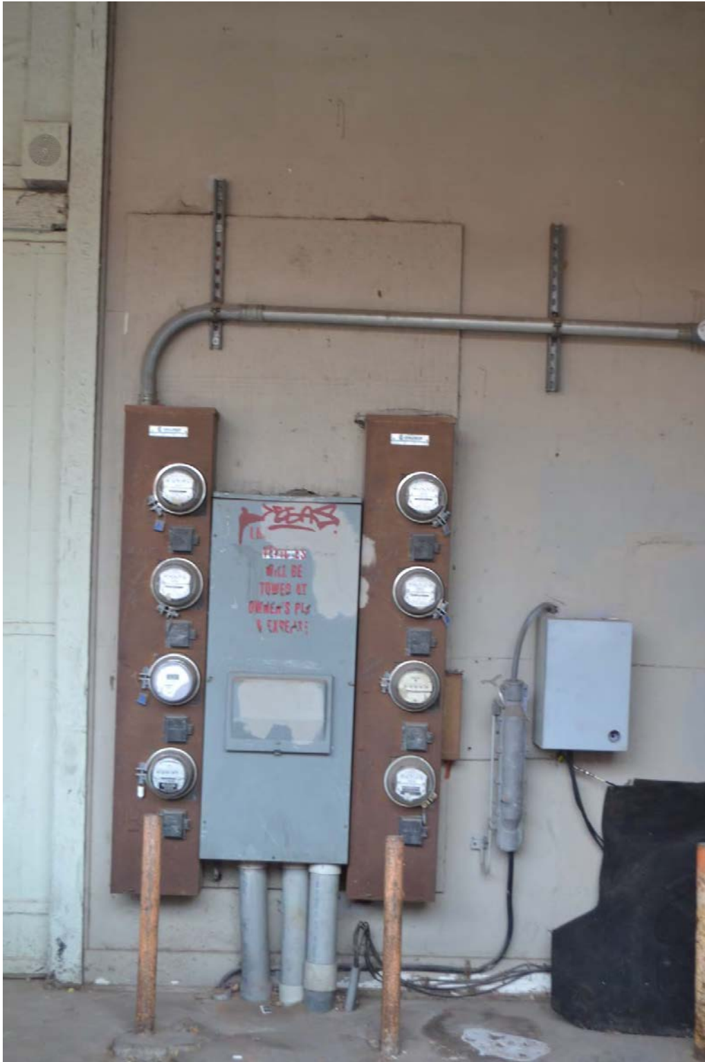
116 E. Jackson Ave. - Utility meters to be hidden with wood slat screen
