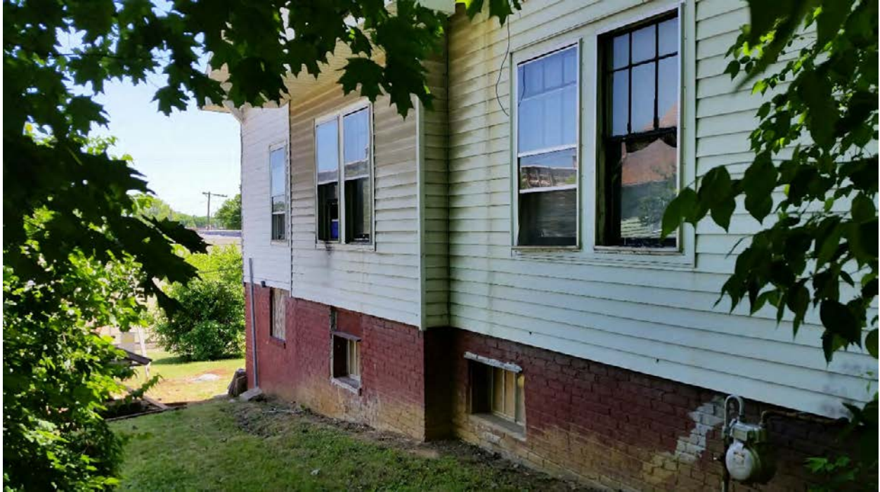
300 E. Oklahoma - Window D on northeast to be replaced
