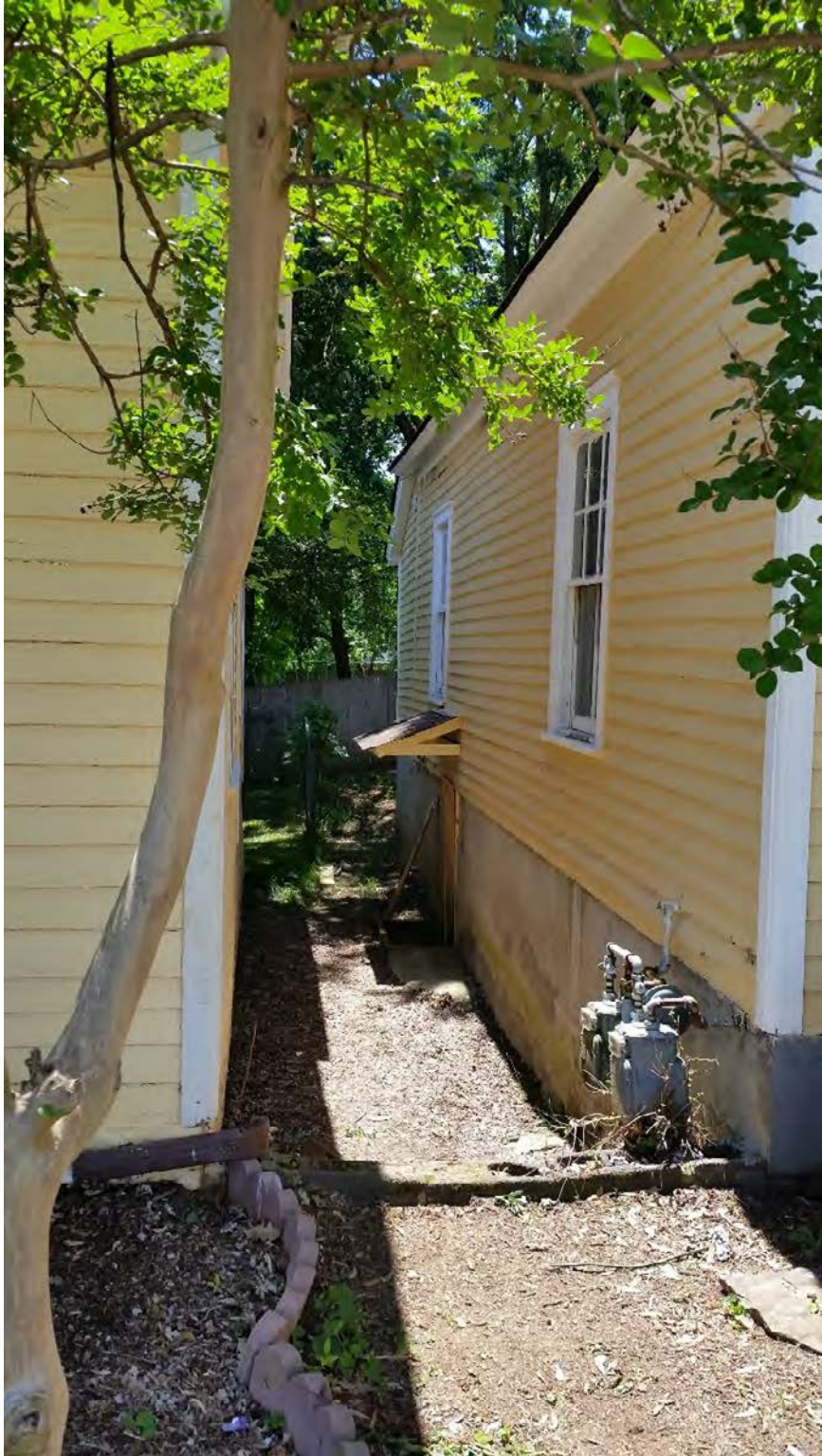
1209 Harvey - South side of house as seen from the street where windows are to be replaced
