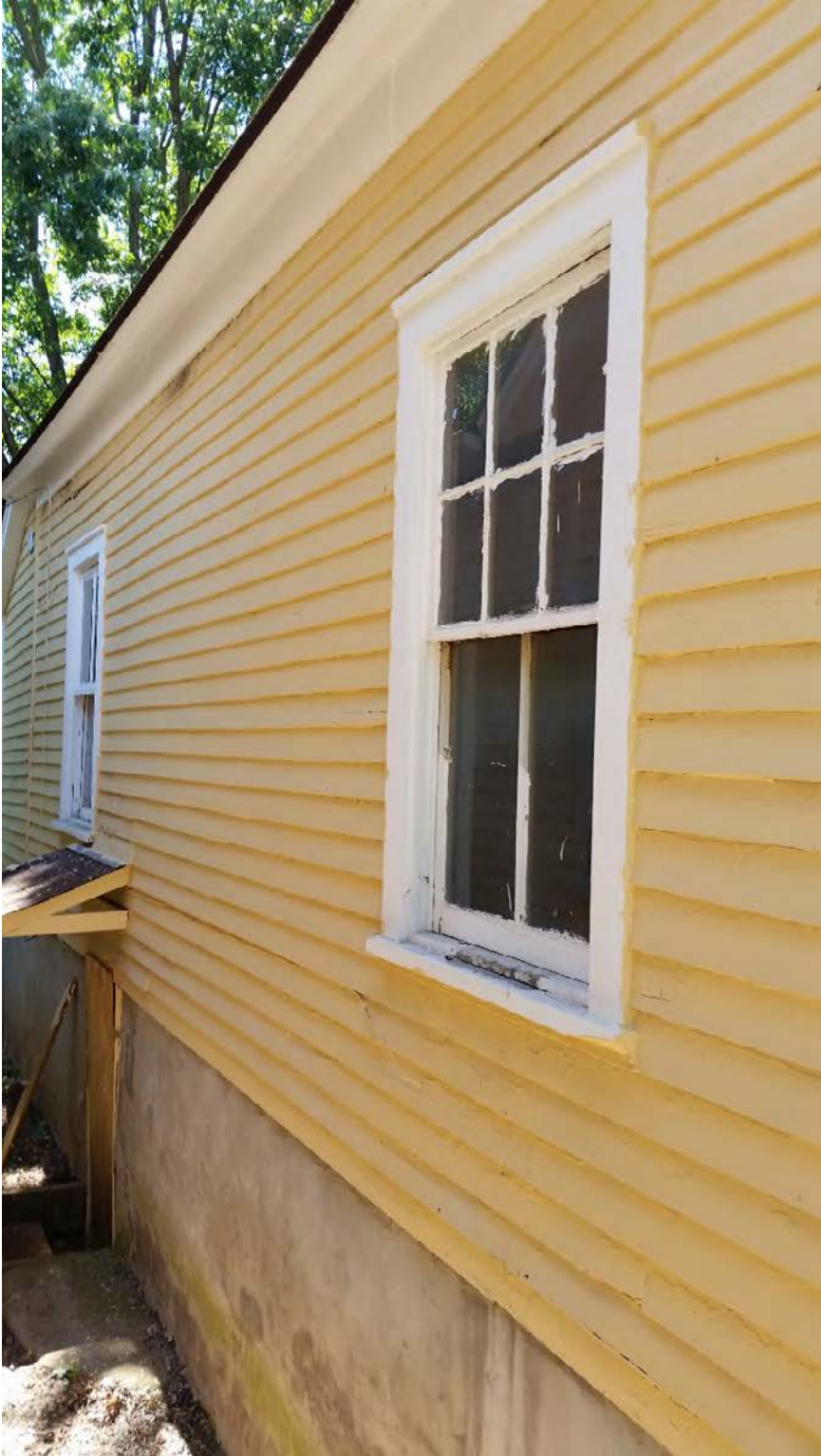
1209 Harvey - Windows on south side to be replaced (closer view)
