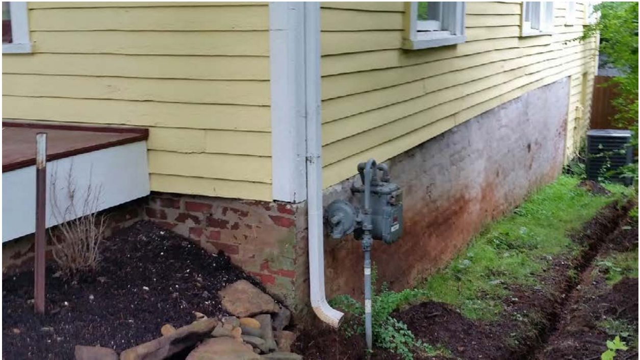
424 E. Oklahoma - Foundation masonry to be repaired
