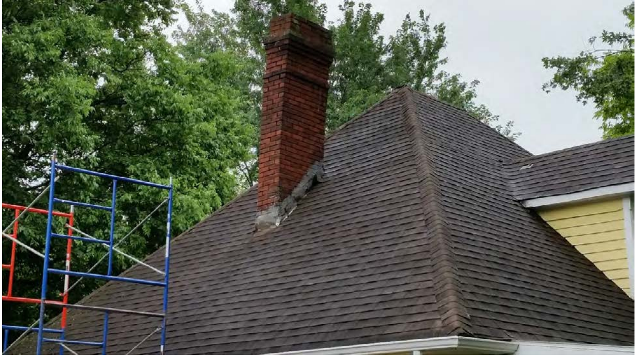
424 E. Oklahoma - Chimney to be rebuilt
