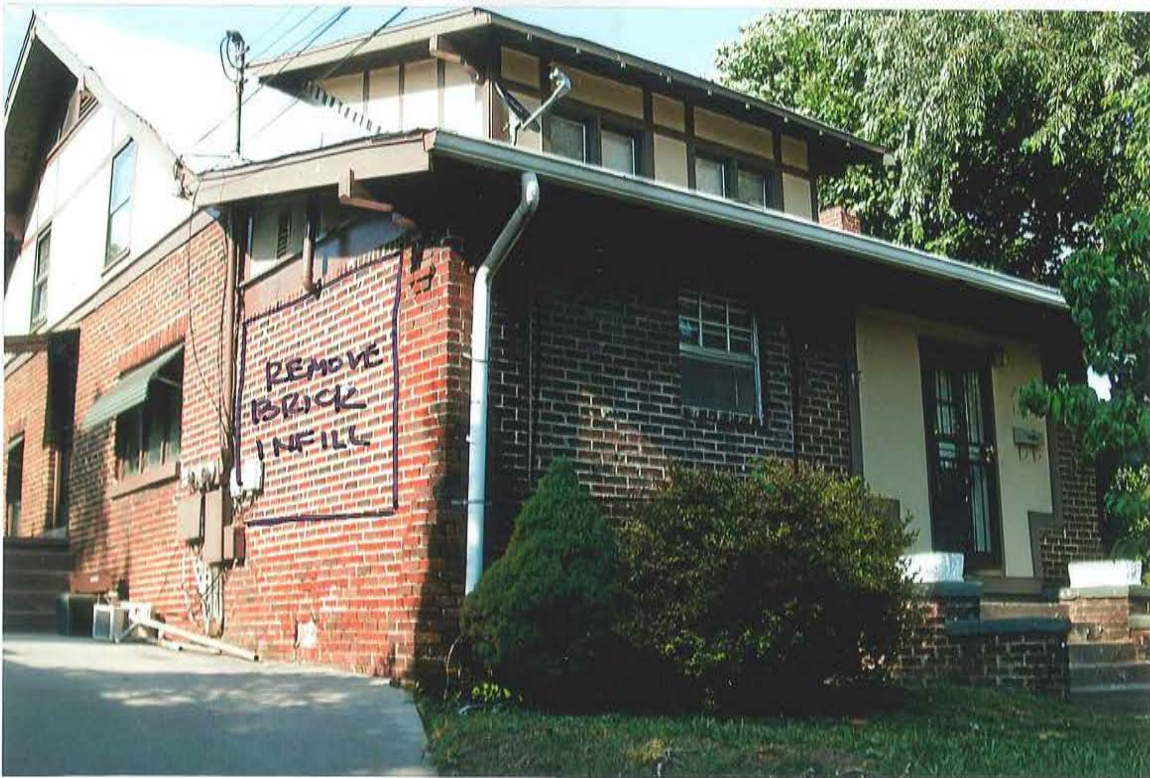
ENCLOSED PORCH (INFILL BRICK TO BE REMOVED)
