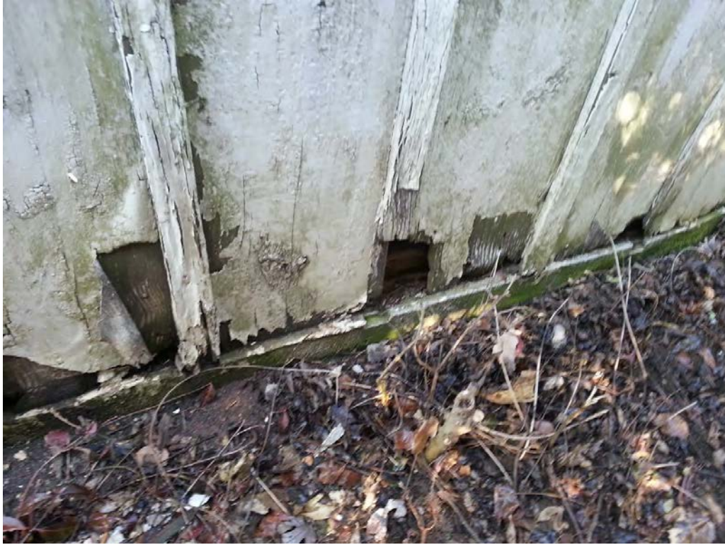
119 W. Glenwood - Siding deterioration at base
