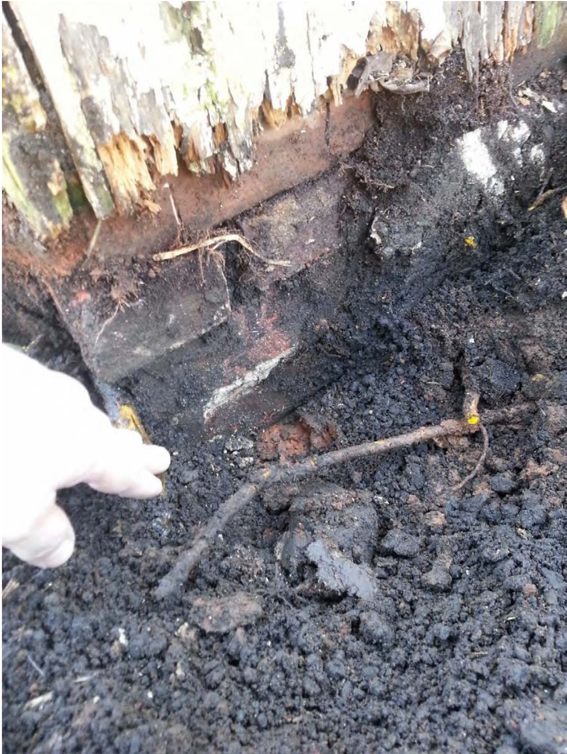
119 W. Glenwood - Foundation rot
