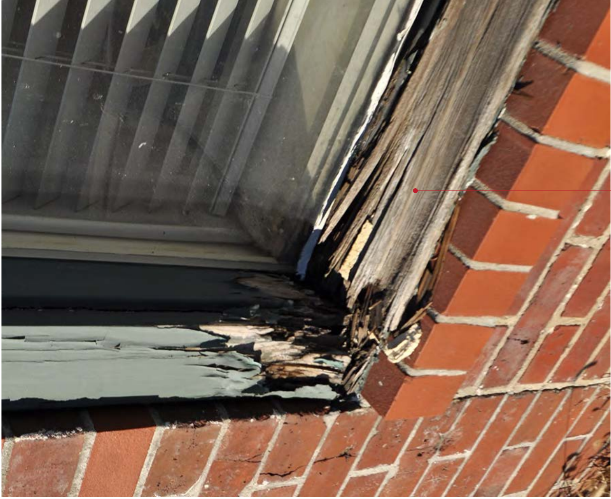
EXISTING WOOD WINDOWS - TYPICAL CONDITIONS
