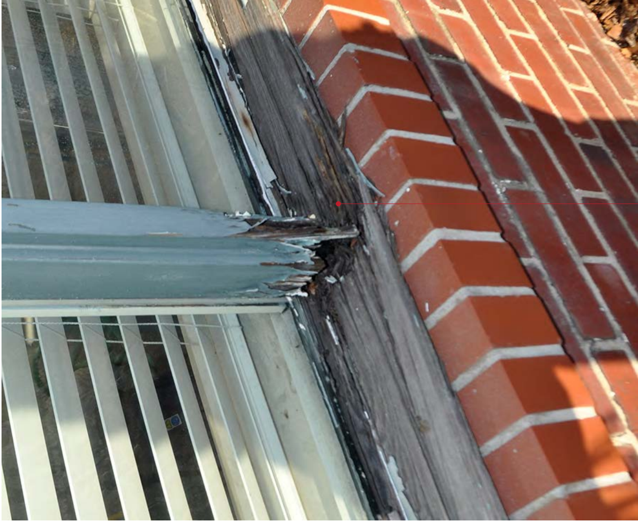
EXISTING WOOD WINDOWS - TYPICAL CONDITIONS
