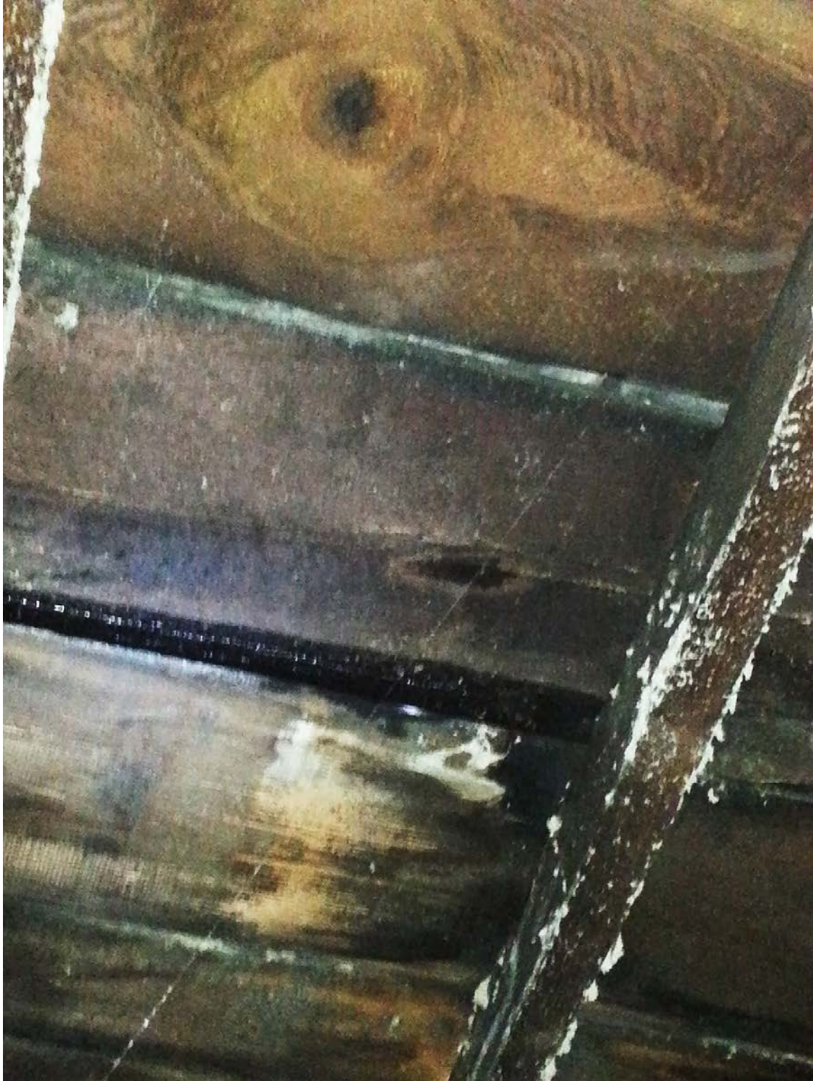
1806 Washington - Rain dripping through wood underlayment
