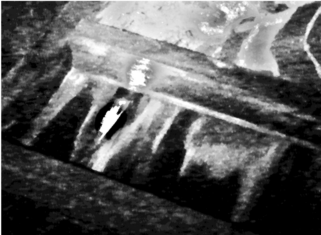
1806 Washington - Daylight showing through hole south of chimney. The hole is 1x4 inches
