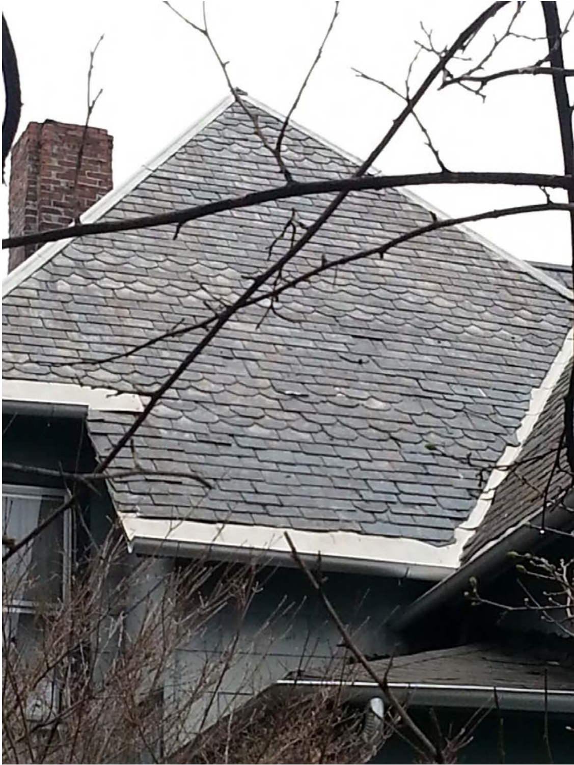
1806 Washington - Rear, from alley, showing missing slates
