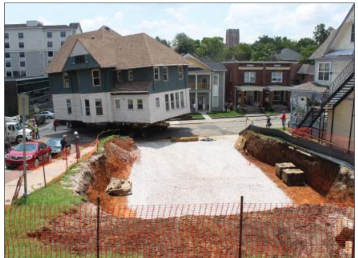
One of three Victorian-style houses was saved from demolition to make way for a new University of Tennessee science building. The house at 1302 White Avenue was moved to 1201 Clinch Avenue in the Fort Sanders neighborhood.
