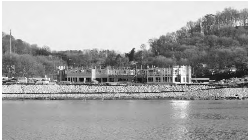
South Waterfront construction continued on the Cityview at River Walk condominiums at the site of a former glove factory on Blount Avenue.
